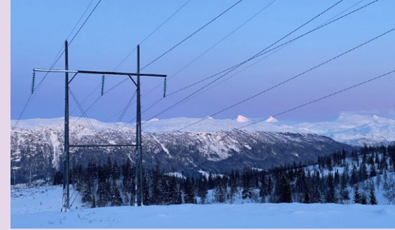
Photo: Statnett SF
